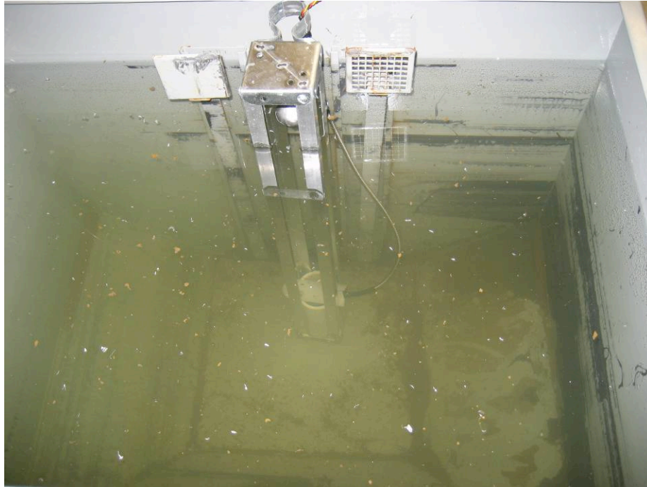
Figure XX: Inside of tank with installed Reed Switch
